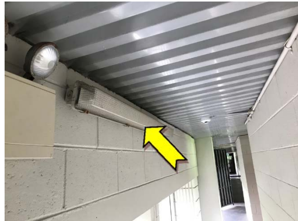
Photo 4. Interior, throughout, fluorescent light fitting - double tube – suspected PCB-containing capacitors.
