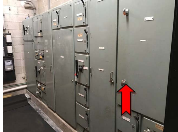
Photo 2. Interior, electrical switch room, electrical backing board – suspected asbestos-containing bituminous backing board.
