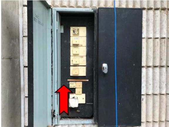
Photo 1. Exterior, west elevation adjacent to main entrance, electrical box – suspected asbestos-containing bituminous backing board.
