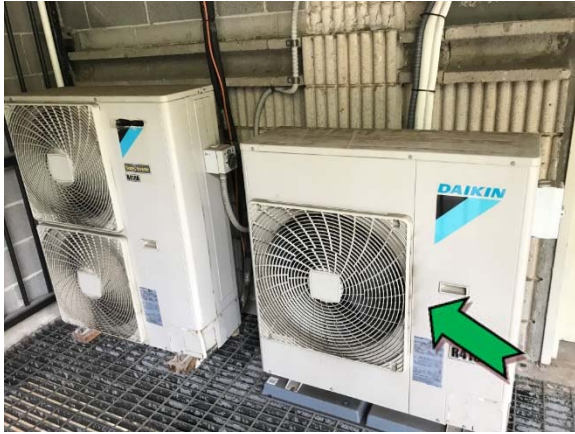
Photo 7. Exterior, west elevation central staircase, air conditioning unit – suspected negative ODS.
