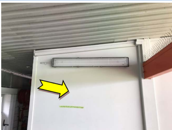
Photo 5. Interior change rooms throughout, walls – suspected lead-containing white upper paint system.
