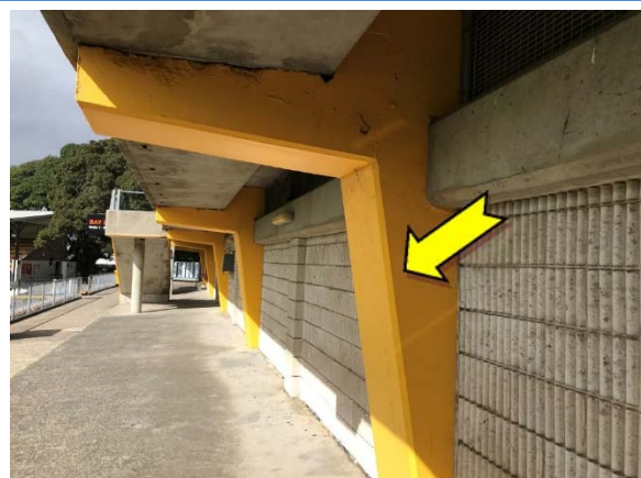
Photo 6. Exterior, throughout, features – suspected lead-containing yellow upper paint system.
